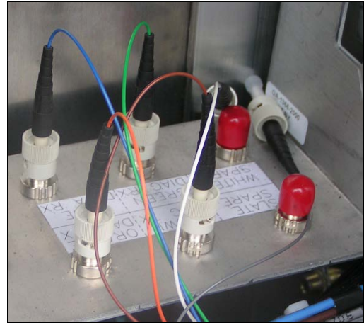
Figure 6: Fiber Patch Panel
